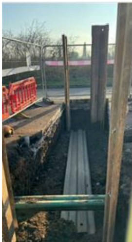
Photo showing fallen sheet pile
