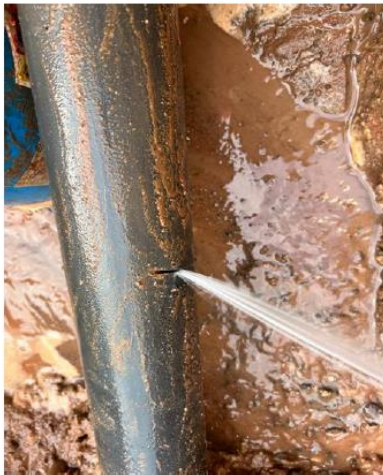
Photo 1: Damage To Pipework
