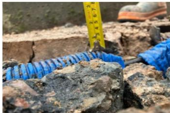
Depth of cable below slab
