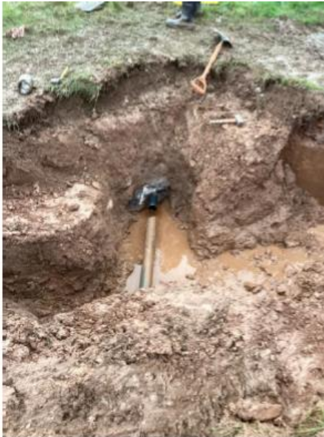
Photo 1: Damaged PVC pipework
