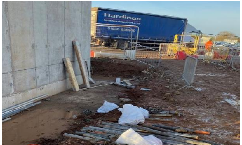
Pic 1: IP was stepping from soft ground onto the concrete blinding
