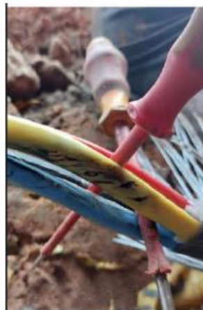
Photo 2: View of removed damaged cable showing compression
