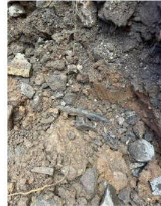
Photo 1: Exposed Cable and stone underneath
