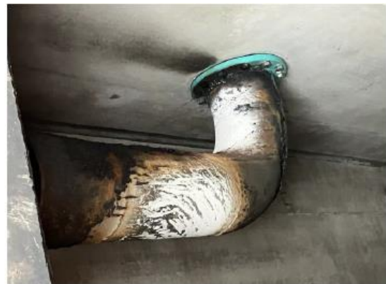
Photo 2: Damage to the internal pipe
